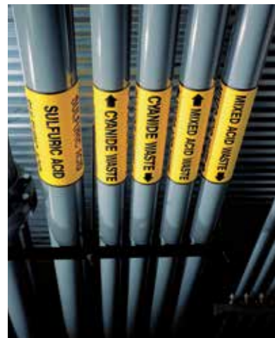
Installed piping for the transport of chemical substances
